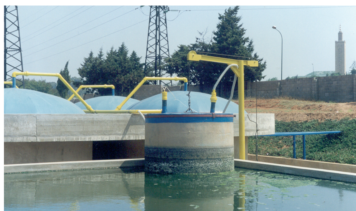
Research - Demonstration installations at partner institutions, here IAV Hassan II
